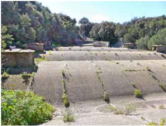
Willis's Magazine: the extensive vaulted roof; there was continuing concern about the site's vulnerability to Spanish shell fire
